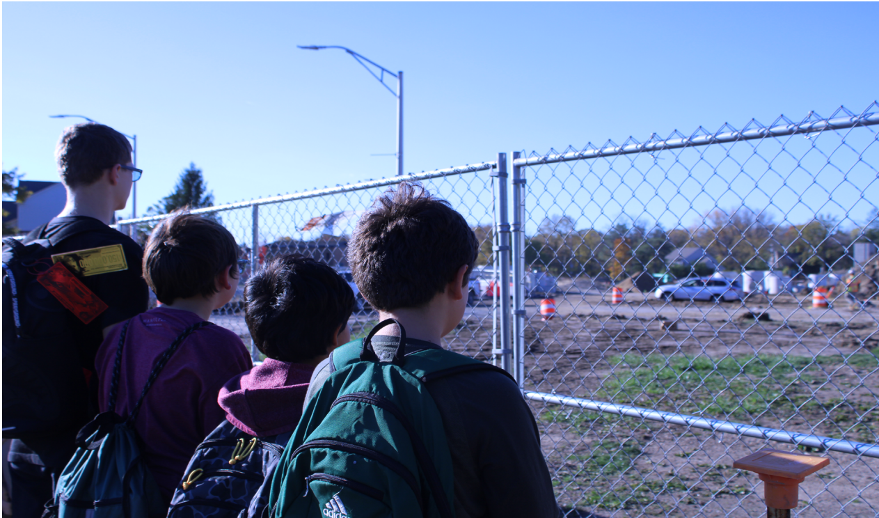
Every day students walk past the new Logan Elementary School being built in front of Clague. The middle school community has adjusted for the construction. This has included new traffic patterns and traveling to other schools for athletic fields. SATVIKA RAMANATHAN
