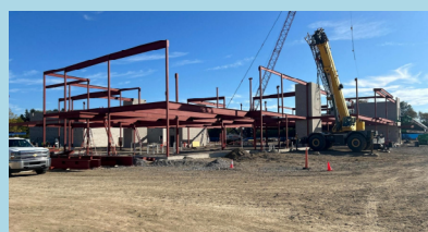
The beginnings of the new Mitchell building. PHOTO COURTESY OF ANDREW CLULEY
