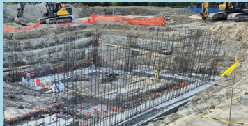
Construction of the basement level concrete footings with wall reinforcing. PHOTO COURTESY OF ANDREW CLULEY
