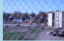
Clague students walk over to see the Logan construction. PHOTOS BY SATVIKA RAMANATHAN
